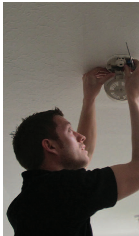
SMOKE ALARM RAISES EARLY WARNING
